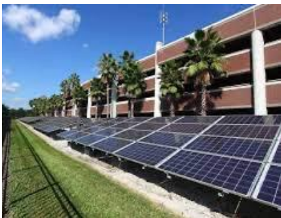
Photovoltaic systems on-site at UCF
